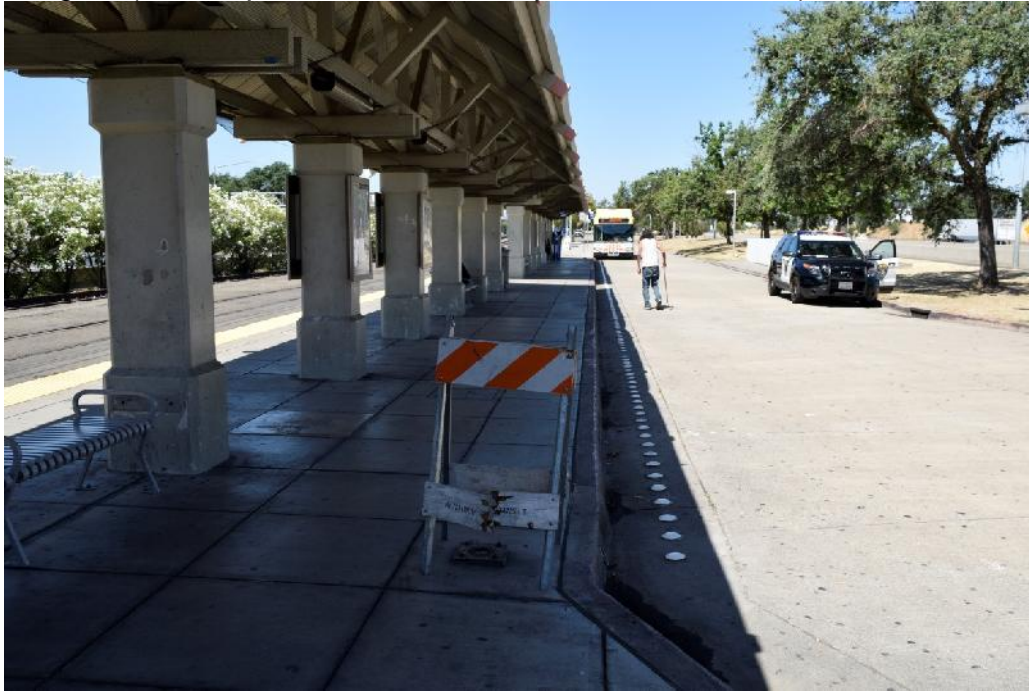
Image 4 (broken pole base covered by broken barricade)
