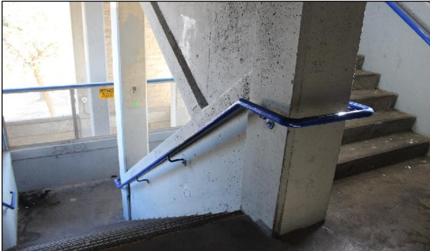
Improving visibility on the stairs was identified as a way to improve safety while transferring.
