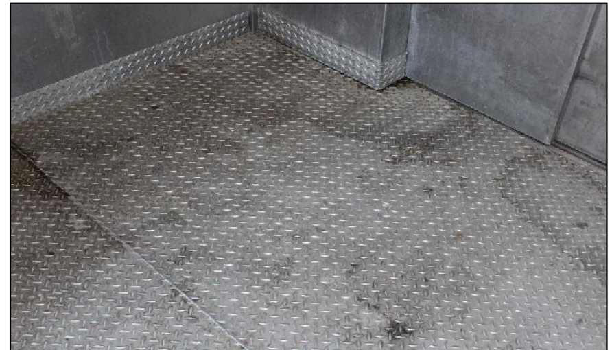
The elevator is unclean and smells due to use as a restroom.
